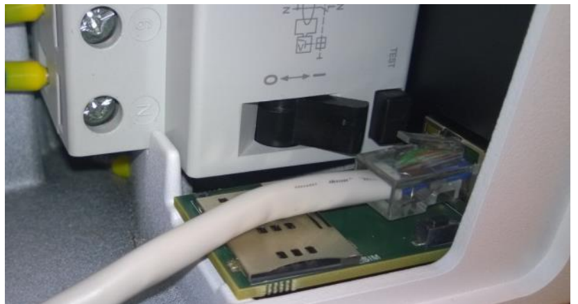
Figure 42: Ethernet UTP cable connected to the connector next to the protection element (RCD in this case)
