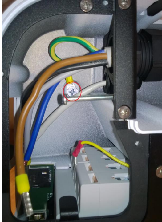
Figure 38: Ground wire secured to the enclosure using the screw
