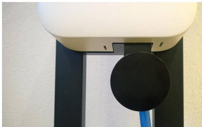
Figure 51: Charging station with installed big metal circle where magnetic cable hand can be attached to
